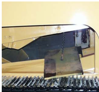
10: Lower existing toggle onto main conveyor. Remove and replace with new toggle plate.
