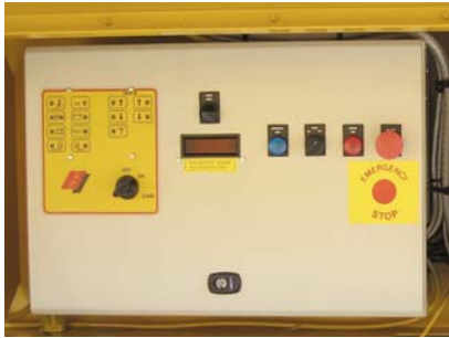
1: Emergency stop and ignition switch in control box
