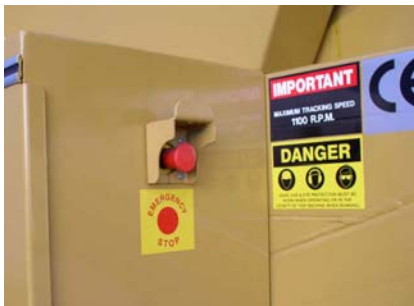
4: Emergency stop on hydraulic box
