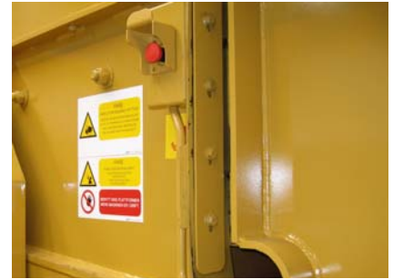
3: Emergency stop on L/H side of crusher box
