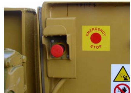
6: Emergency stop on R/H side of crusher box
