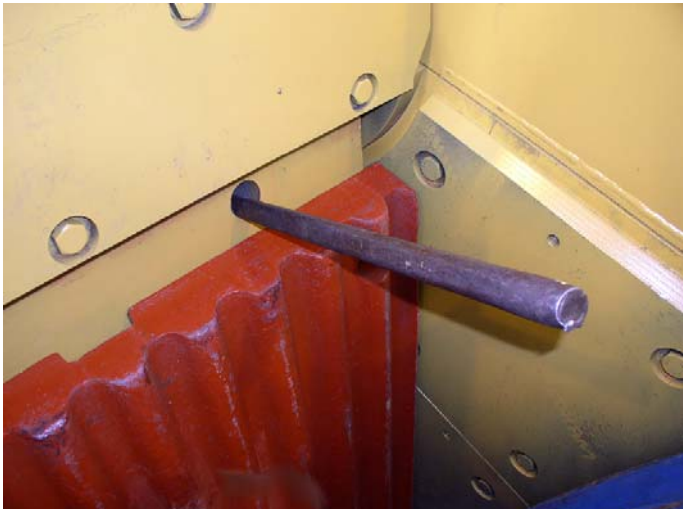
11: Place a suitable bar in hole to help with lining up the wedge.
