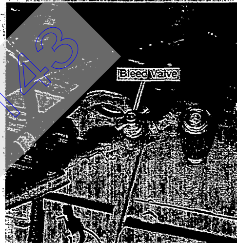
Bleed Valve at Converter
